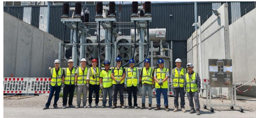
The successful energization of PF1 converter transformer (66 kV)
