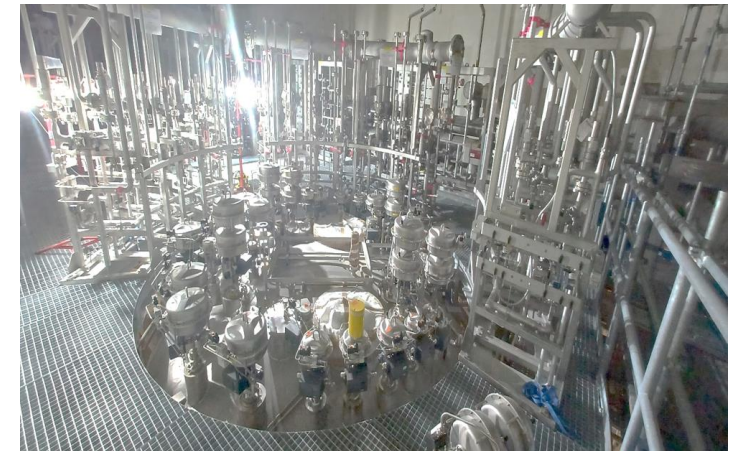
ACB top platform with warm panels and valve actuators installed
